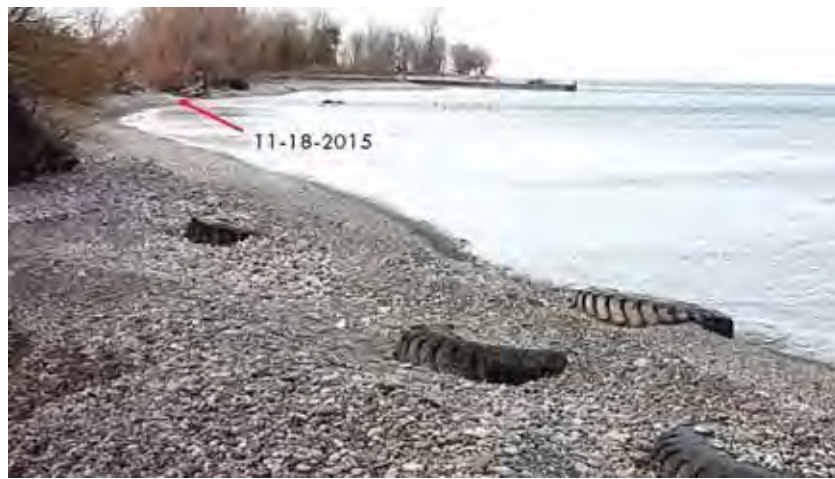
Location of the breach in Nov. 2015 (~WL 244.5 IGLD85)
