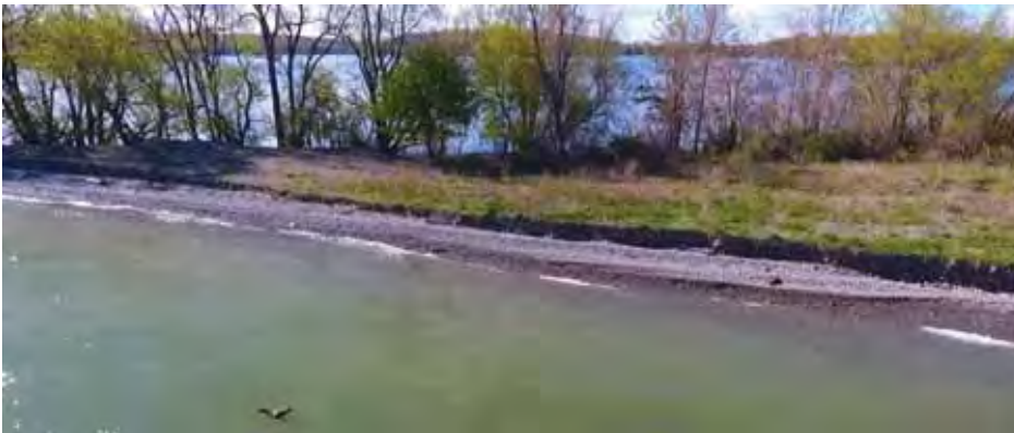
West side of the breach looking south, May 10, 2017 (drone view) (WL~248.6)
