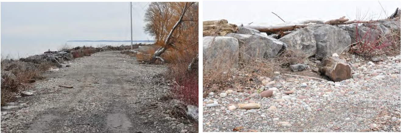
Figure 4-4 (Left) Low areas of the west barrier bar access road subject to flooding and erosion. (Right) Typical erosion occurring immediately inboard of the stone armoring the lake side of the west barrier bar.
